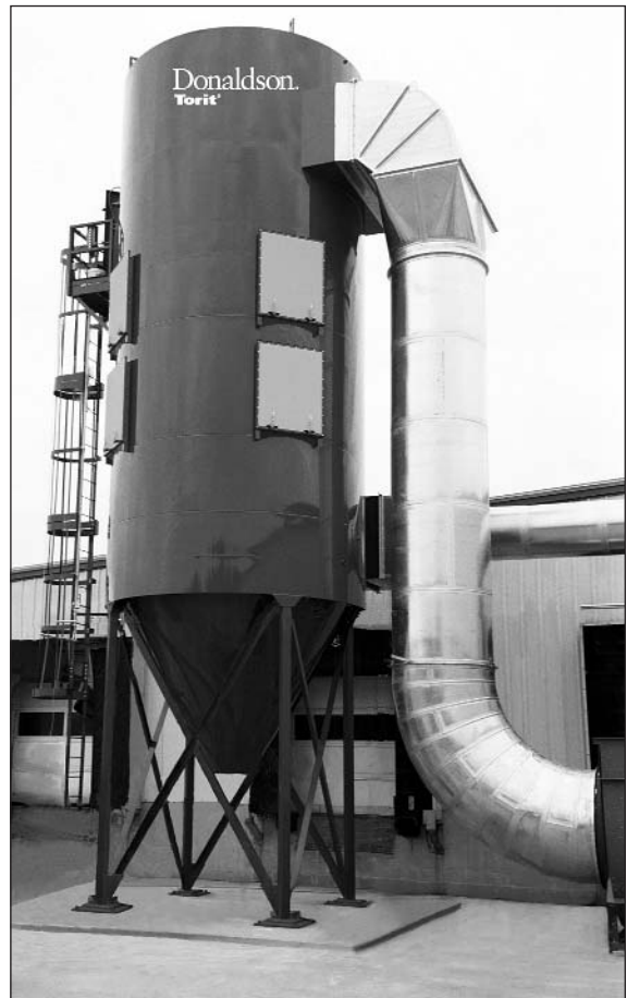
RF Baghouse Collector
